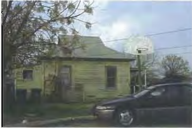
PHOTO 1 Dilapidated residence on Ivy Avenue. APN 477 113 06 08660 KG
