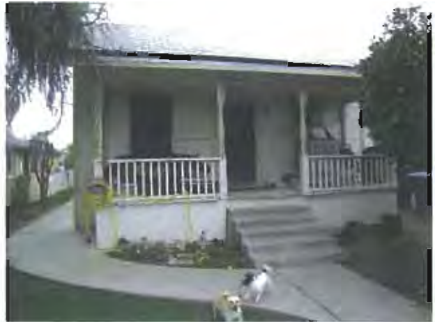
PHOTO 34 Dilapidated residence APN 467 172 13 1527 AY
