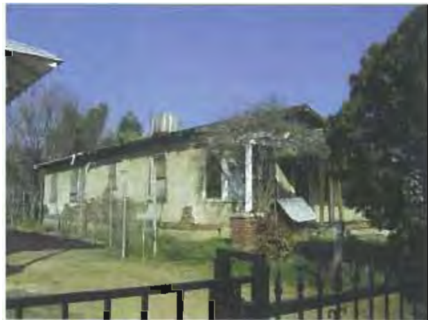
PHOTO 55 Dilapidated residence with foundation, roof and exterior walls in need of repair. APN 465 193 10 0071 JL
