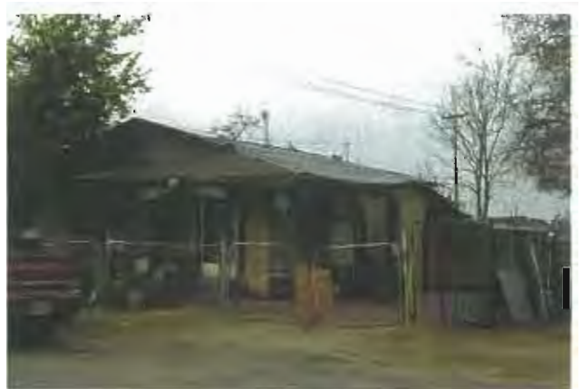
PHOTO 4 Dilapidated residence on Eunice Avenue. APN 477 114 23 08662 KG
