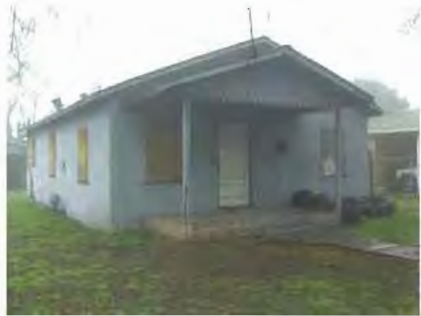
PHOTO 76 Dilapidated residence on Atchison Street. APN 478 252 08 1502 AY
