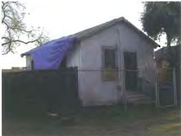
PHOTO 39 Dilapidated residence on Oleander Ave. APN 465 171 17 1577 AY
