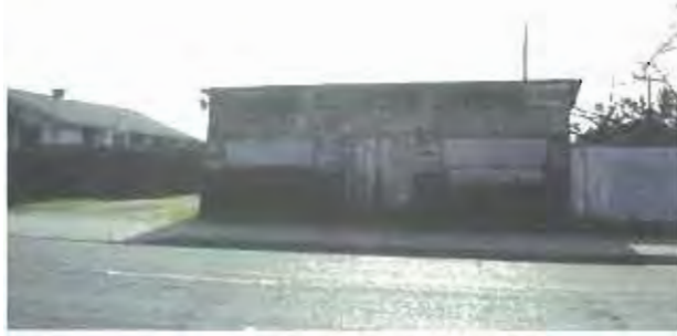
PHOTO 77 Dilapidated, abandoned commercial building on Modoc St. APN 4641 111 04 8709 KG
