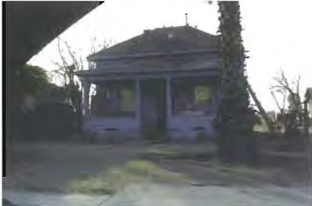
PHOTO 73 Dilapidate residence on Woodward Avenue. APN 328 150 36 08739 KG
