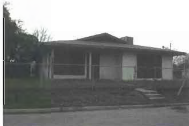
PHOTO 16 Deteriorated residence on Santa Clara Street. APN 477 114 06 08665 KG
