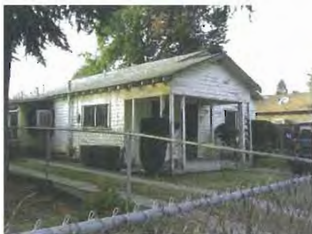
PHOTO 47 Dilapidated residence with deteriorated siding and a foundation in need of repair. APN 478 261 15 0028 JL
