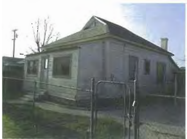
PHOTO 38 Dilapidated residence on Tupman Ave. APN 465 172 08 1573 AY
