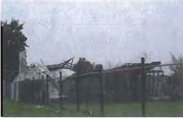
PHOTO 5 Dilapidated and collapsed building on A Street. APN 458 230 24 8678 KG
