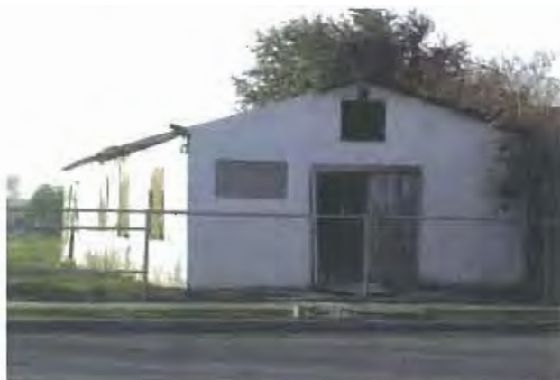
PHOTO 46 Dilapidated storage building on Thorne Avenue. APN 8737 KG
