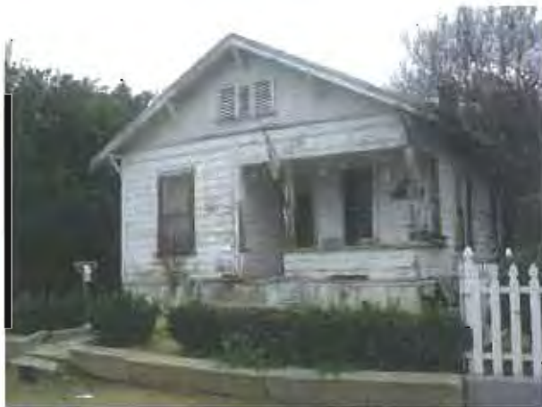
PHOTO 3 Dilapidated residence with failing foundation on Stanislaus Street. APN 467 166 15 08626 KM
