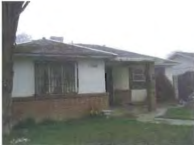
PHOTO 49 Dilapidated residence on Ivy Avenue. APN 478 252 17 0031 JL
