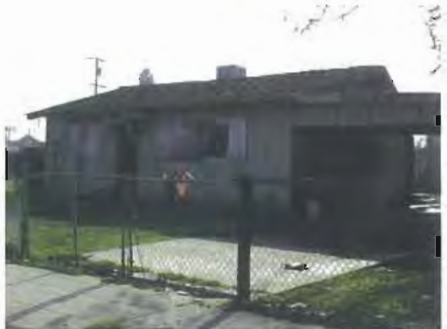
PHOTO 42 Dilapidated residence. APN 464 171 03 1614 AY
