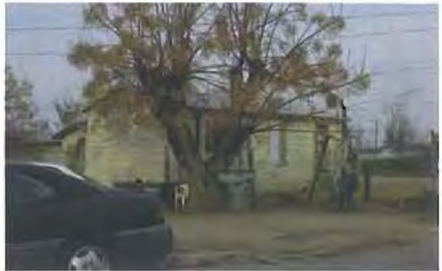
PHOTO 2 Dilapidated residence on Eunice Ave. APN 477 113 05 08661 KG
