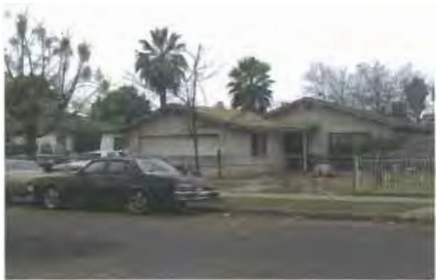
PHOTO 27 Dilapidated residence with a broken garage door and foundation in need of repair. APN 478 240 29 1517 AY
