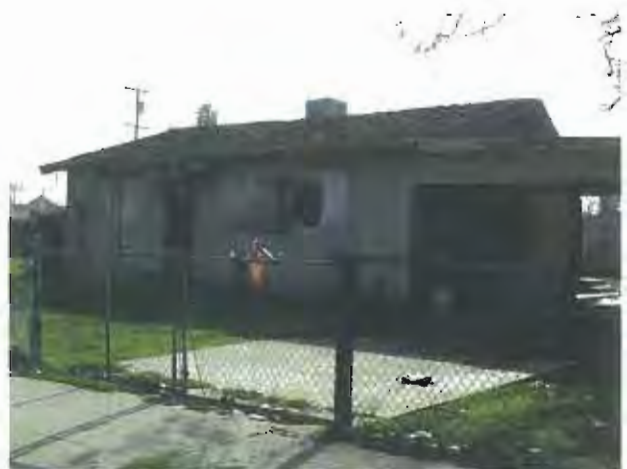
PHOTO 42 Dilapidated residence. APN 464 171 03 1614 AY
