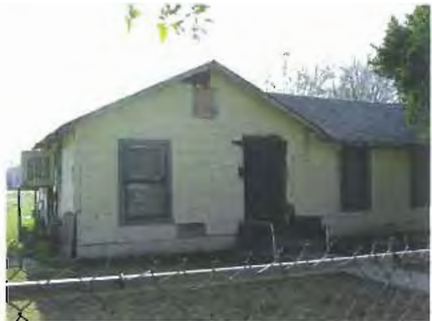
PHOTO 56 Dilapidated residence with asbestos siding, damaged walls and foundation, and a substandard addition on C Street. APN 464 191 06 0073 JL
