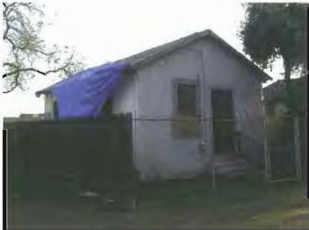
PHOTO 39 Dilapidated residence on Oleander Ave. APN 465 171 17 1577 AY
