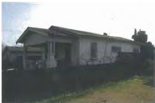
PHOTO 45 Dilapidated residence on Almy Ave. APN 465 216 04 1566 AY
