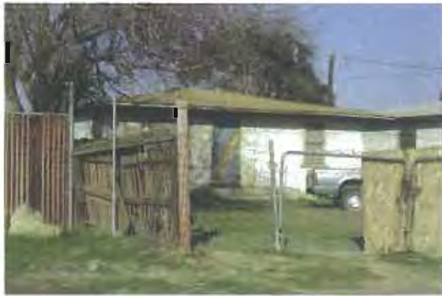
PHOTO 21 Deteriorated residence on Valencia Avenue. APN 329 161 22 08748 KG
