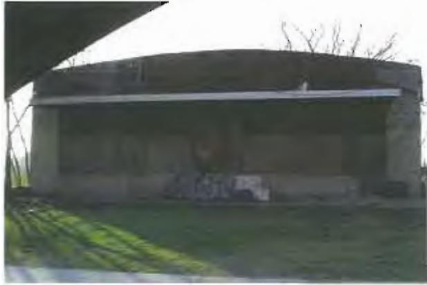
PHOTO 57 Dilapidated commercial building APN 326 150 036 8740 KG
