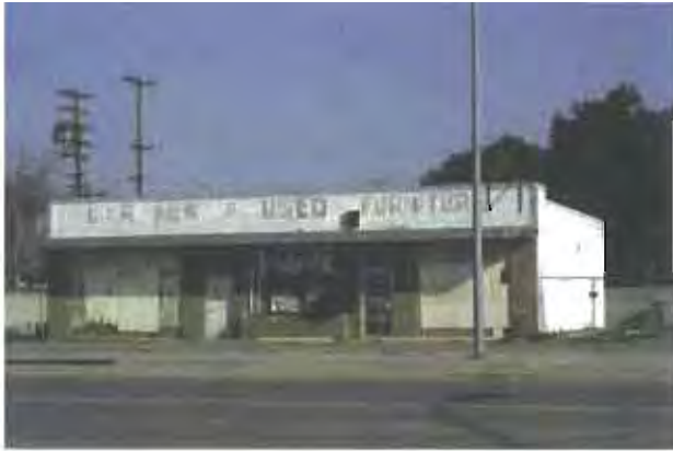
PHOTO 65 Dilapidated commercial building. APN 479 211 10 8746 KG
