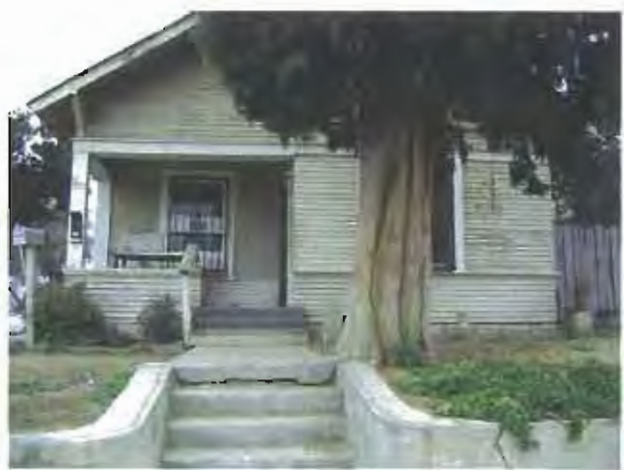
PHOTO 54 Dilapidated residence with foundation and retaining wall in need of repair on Tupman Avenue. APN 467 165 16 0050 JL
