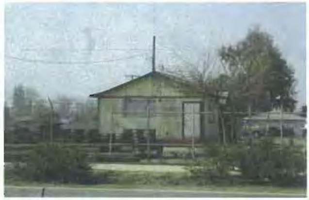
PHOTO 58 Deteriorated commercial/industrial building with open storage and unpaved parking on Stanislaus Street. APN 328 150 38 8723 KG
