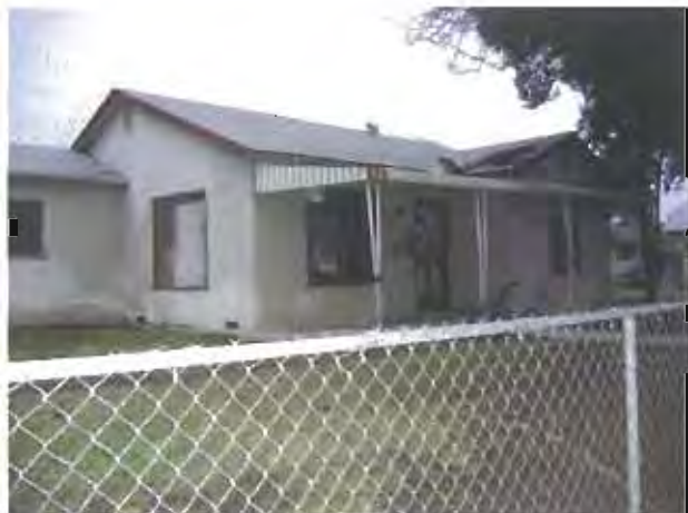
PHOTO 67 Dilapidated residence with a porch of substandard construction, and cracks and holes in the exterior walls on Martin Luther King Jr. Boulevard. APN 467 233 01 0043 JL
