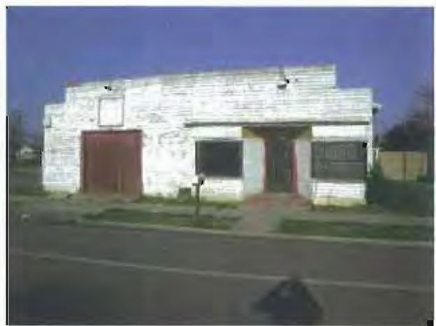
PHOTO 68 Dilapidated, obsolete commercial building with structural problems (walls of the building appear to be leaning) on Bardell Avenue. APN 465 172 15 1574 AY
