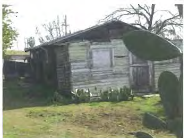
PHOTO 88 Dilapidated residence on Holly Avenue. APN 465 232 13 1563 AY
