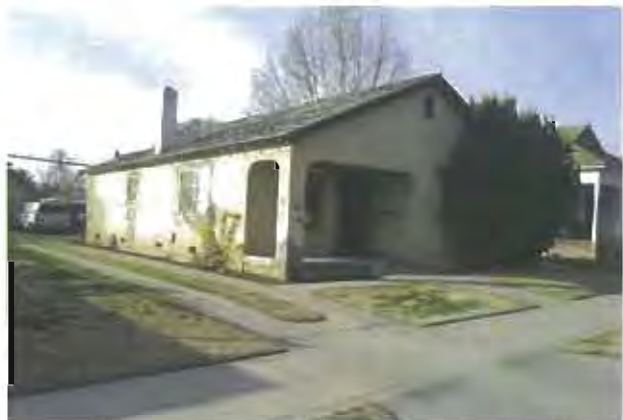
PHOTO 23 Deteriorated residence on California Ave. APN 478 201 12 1464 AY
