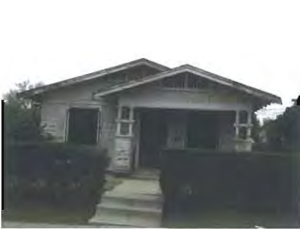
PHOTO 37 Dilapidated residence on Elm Avenue. APN 467 192 10 1543 AY
