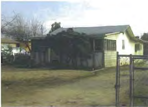
PHOTO 11 Dilapidated residence APN 477 134 04 08614 KM
