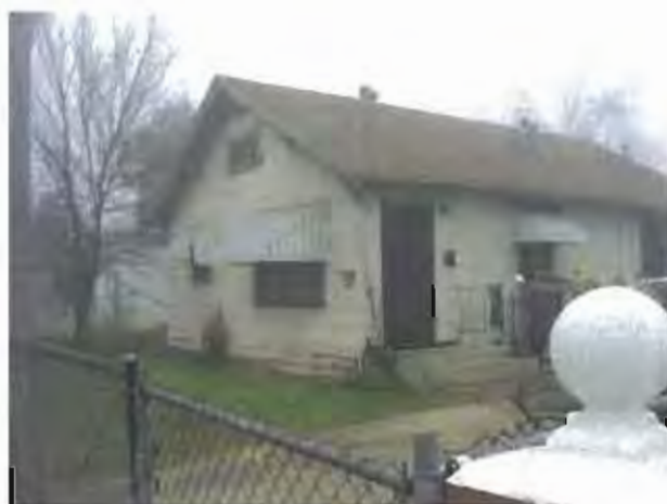
PHOTO 48 Dilapidated residence with foundation and exterior siding in need of repair on Ivy Avenue. APN 478 133 15 0030 JL
