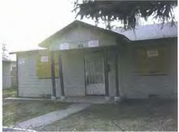
PHOTO 90 Dilapidated, boarded up residence on Ivy Avenue. APN 478 261 16 0027 JL
