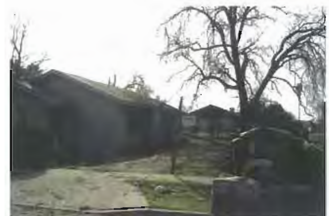
PHOTO 28 Dilapidated residence on Lotus Avenue. APN 464 121 33 08707 KG
