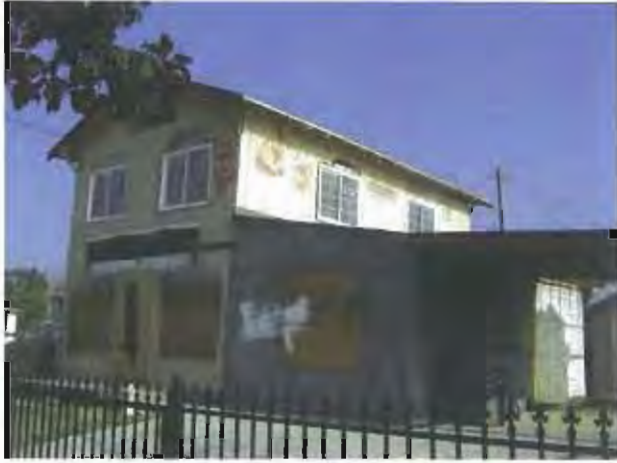
PHOTO 69 Dilapidated residence on C Street. APN 465 213 15 0067 JL
