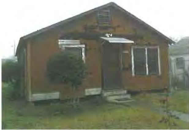
PHOTO 29 Dilapidated residence lacking a proper foundation and with walls in need of repair on Lorena Avenue APN 478 182 24 1501 AY
