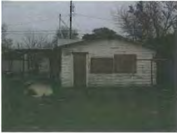
PHOTO 85 Dilapidated, boarded-up residence. APN 467 184 14 1521 AY
