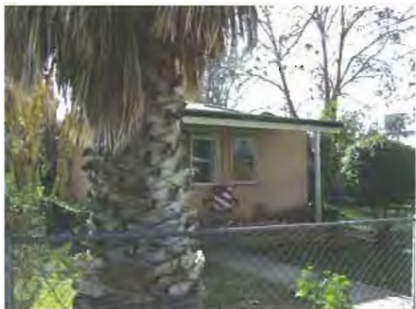
PHOTO 25 Dilapidated residence with tar paper roof and missing window on Inyo Street. APN 464 192 05 0074 JL
