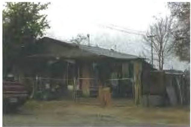
PHOTO 4 Dilapidated residence on Eunice Avenue. APN 477 114 23 08662 KG
