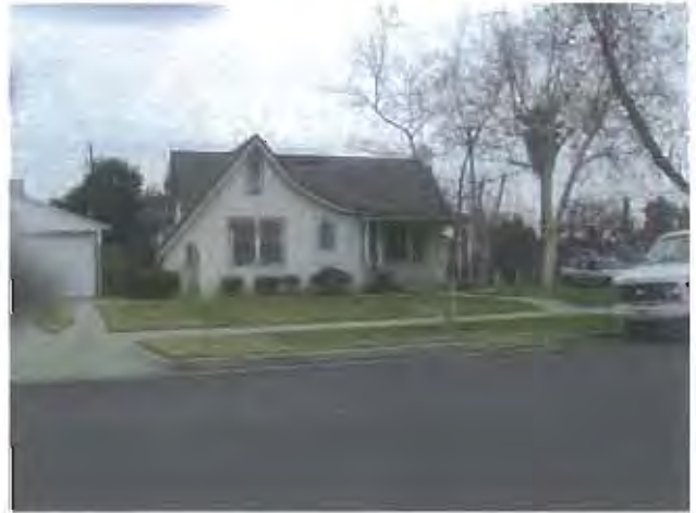
PHOTO 30 Dilapidated residence with deteriorated roof and failing foundation on Calaveras Avenue. APN 467 213 08 8627 KM
