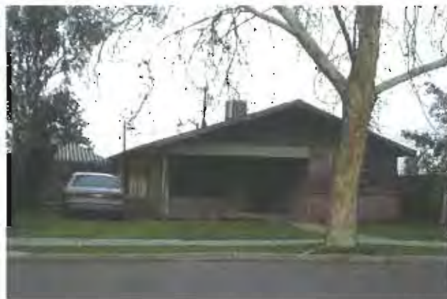
PHOTO 19 Deteriorated residence on C Street. APN 465 125 15 08694 KG
