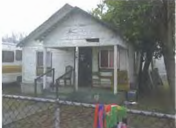
PHOTO 26 Dilapidated residence with windows, siding and roofing in need of repair on Lorena Avenue. APN 478 182 23
