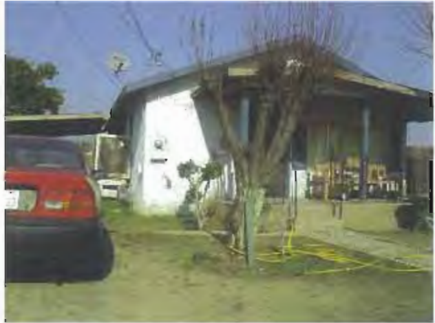
PHOTO 6 Dilapidated residence with unpaved parking area on B Street. APN 328 171 19 8630 KM
