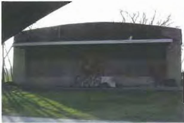
PHOTO 57 Dilapidated commercial building APN 326 150 036 8740 KG
