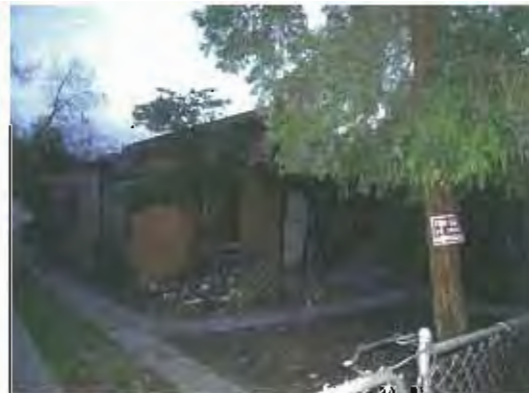
PHOTO 84 Fire-damaged dilapidated residence on Lotus Ave. APN 478 082 20 1480 AY
