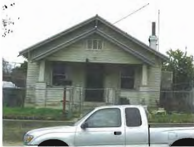
PHOTO 53 Dilapidated residence with a foundation in need of repair on Tupman Avenue. APN 467 165 11 0047 JL
