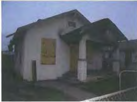
PHOTO 83 Fire-damaged dilapidated residence APN 478 083 32 1473 AY
