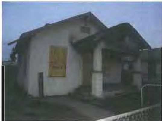
PHOTO 83 Fire-damaged dilapidated residence APN 478 083 32 1473 AY
