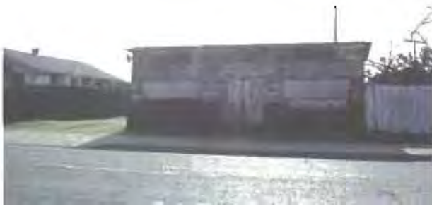
PHOTO 77 Dilapidated, abandoned commercial building on Modoc St. APN 4641 111 04 8709 KG
