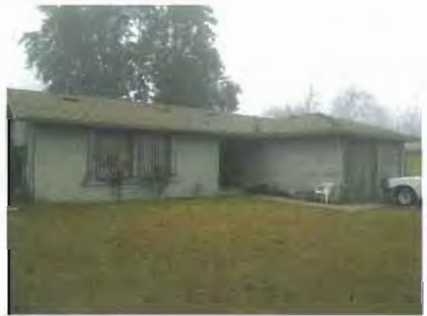
PHOTO 32 Dilapidated residence on Elm Avenue. APN 478 311 23 1505 AY
