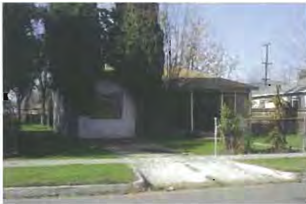
PHOTO 75 Dilapidated residence on Teilman Avenue. APN 479 211 10 08744 KG
