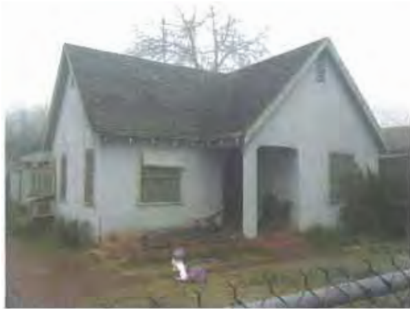
PHOTO 31 Dilapidated residence on Atchison Avenue. APN 478 253 12 1504 AY
