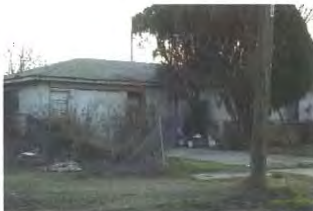
PHOTO 18 Dilapidated residence on Florence Avenue. APN 328 252 12 08742 KG
