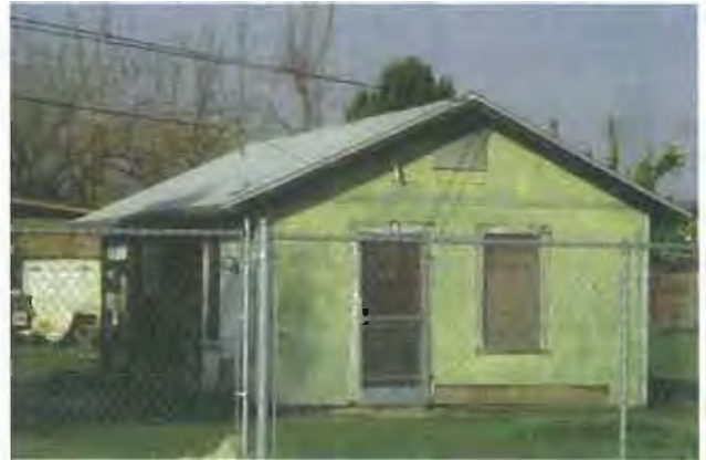
PHOTO 10 Dilapidated residence with asbestos shingle siding and no foundation. APN 477 134 17 8650 KG
