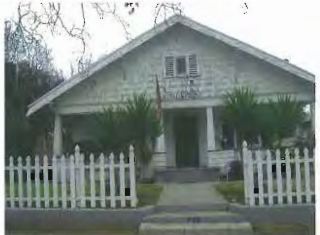
PHOTO 12 Dilapidated residence with failing foundation. APN 467 166 14 08625 KM
