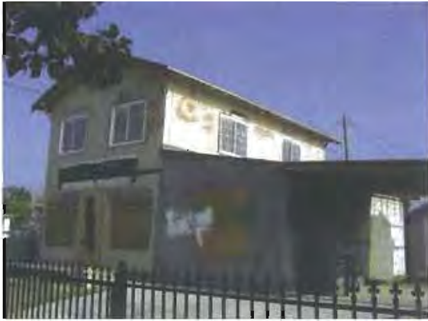
PHOTO 69 Dilapidated residence on C Street. APN 465 213 15 0067 JL
