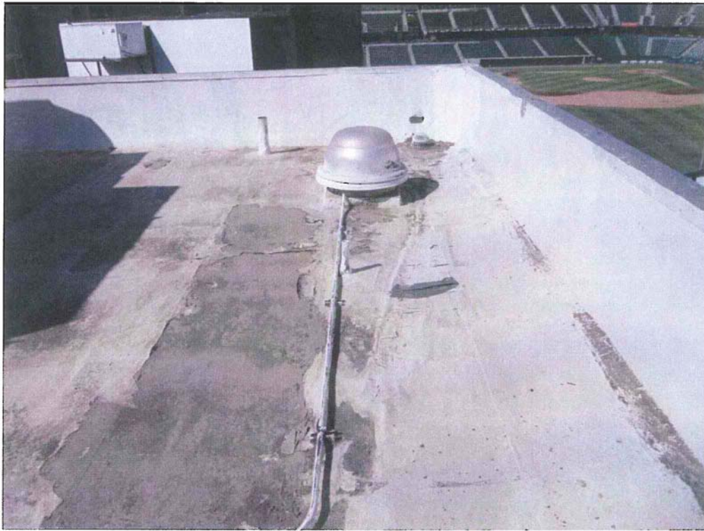
Photograph Number 9 Vent at Corner of Roof Obstructing Drainage
