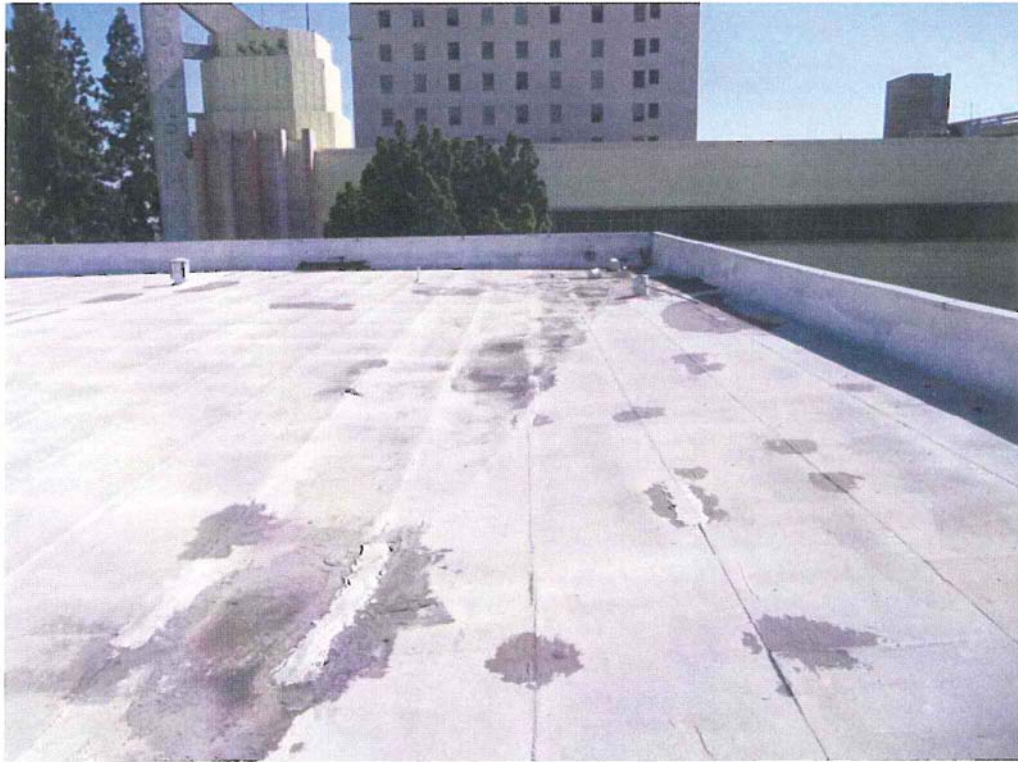
Photograph Number 1 View of Large Cricket and Split Repairs
