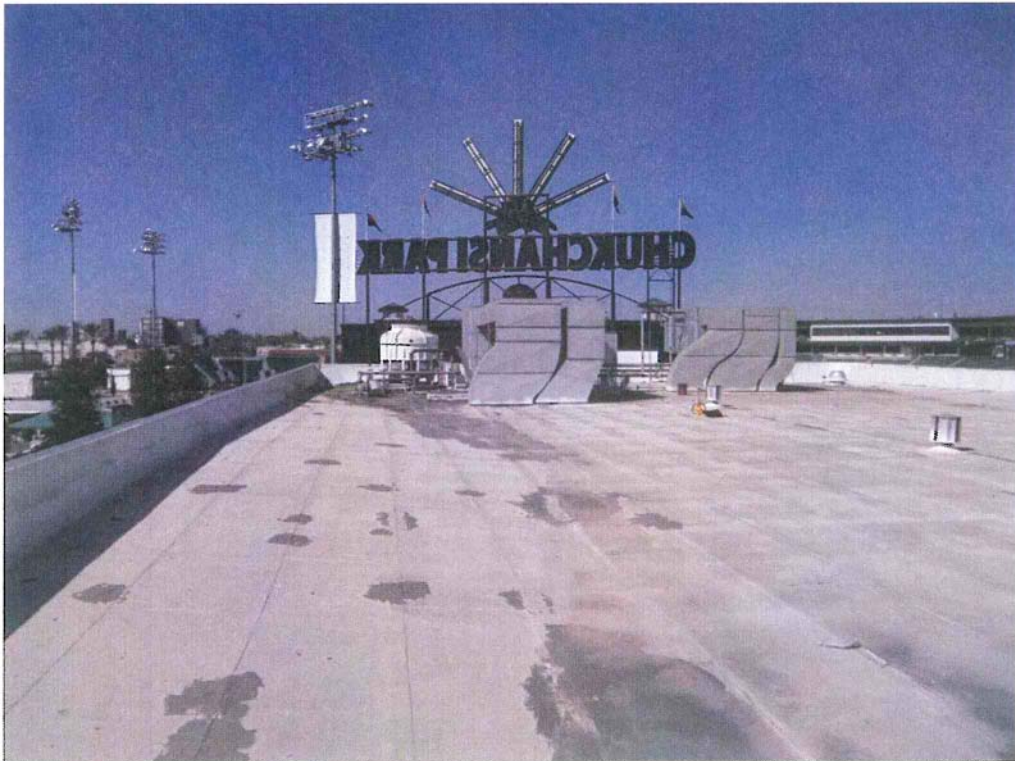
Photograph Number 2 View of Mechanical Equipment at West End of Roof
