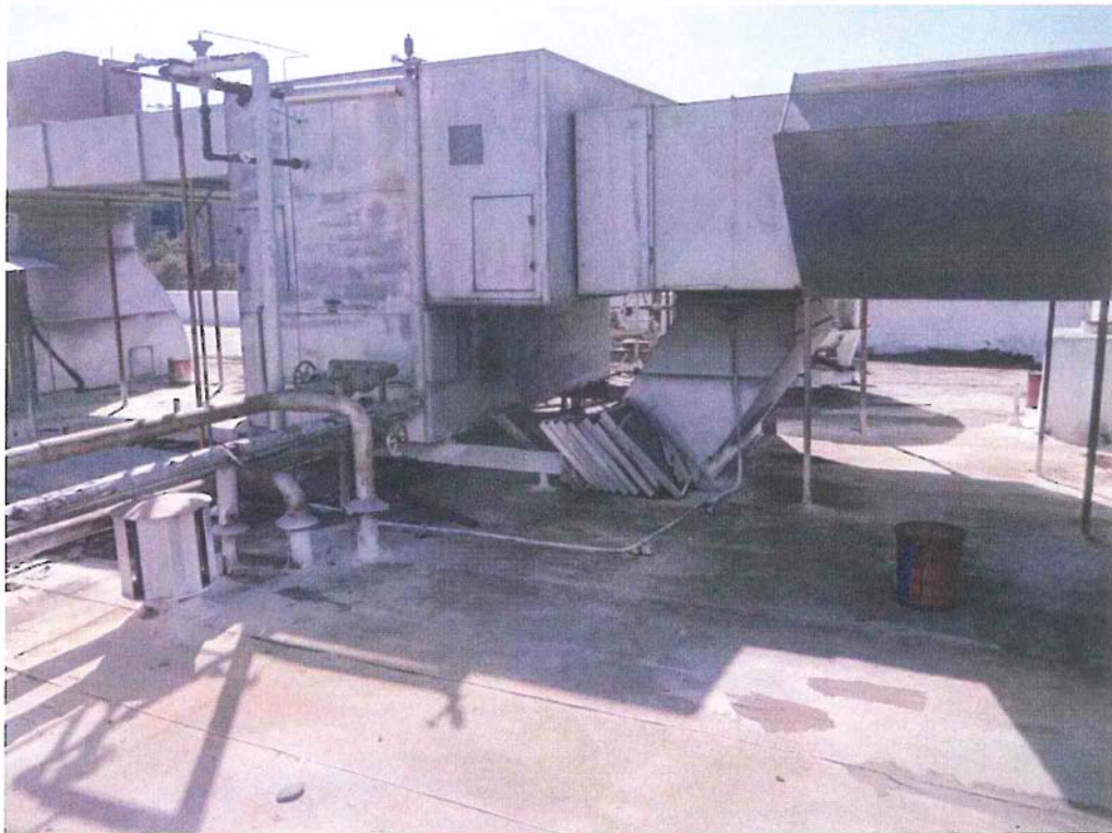
Photograph Number 10 Large Air Handling Unit
