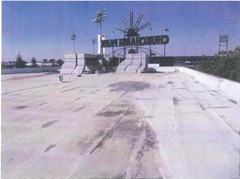
Photograph Number 3 View of Ponding Areas and Field Repairs
