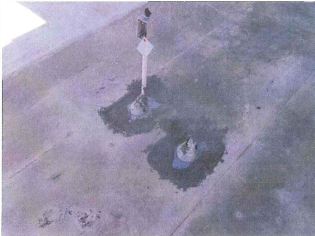
Photograph Number 11 Penetration Flashing Not Incorporated into Roof System
