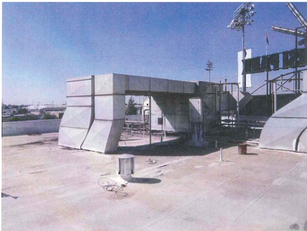
Photograph Number 8 Mechanical Equipment Area
