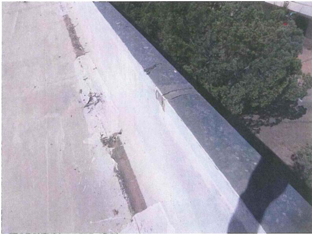
Photograph Number 5 Failed Coping Joint and Repair at Base of Wall
